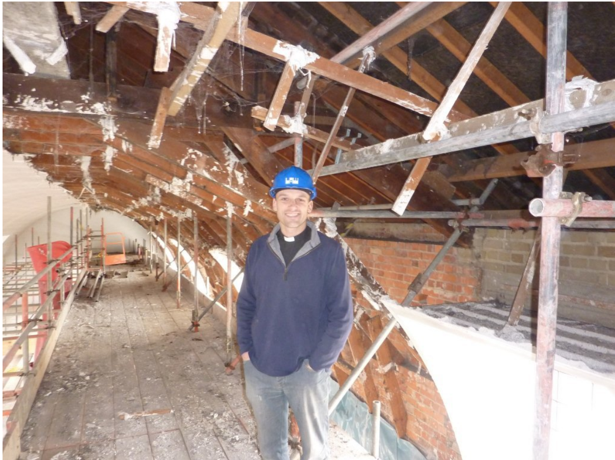
Vicar, Paul Cowan stood by the south side of the ceiling which has been removed and with scaffolding props in place ready for the PV installations to begin.
