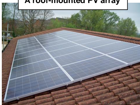
A roof-mounted PV array
